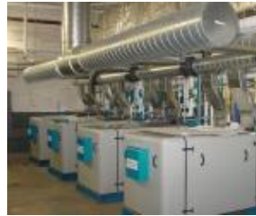
CHP with Boiler
